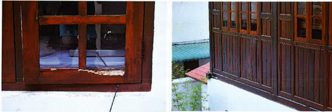
Photo 15: Damages suffered by windows as a result of termite attacks and warping Source: Sanitary Board Conservation Project, Taiping, Perak, 2008
