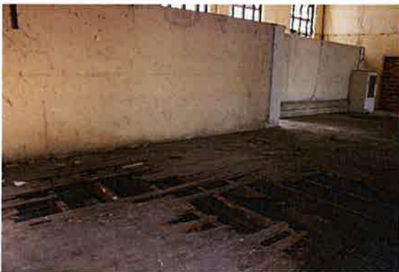
Photo 11: Damaged wood caused by termite attack and wood rot Source: Old Post Office Conservation Works Project, Ipoh, Perak, 2009
