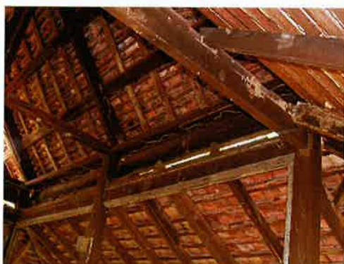
Photo 2: Termite attacks on the roof frame Source: Penghulu Natar House Rehabilitation Project, Merlimau, Melaka, 2009
