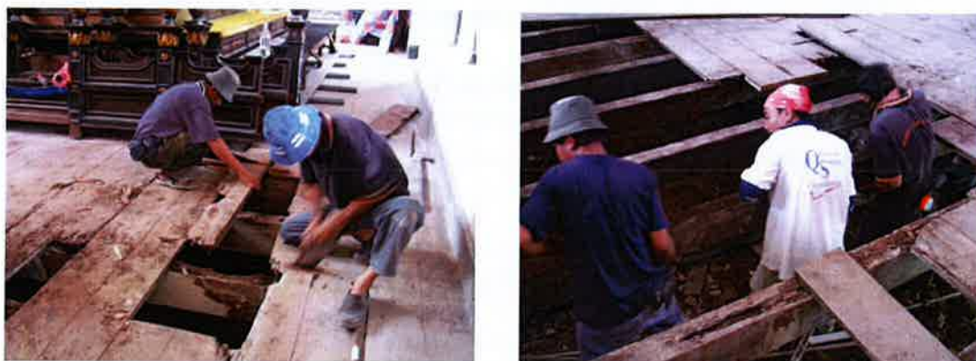
Photo 12: The main damage to the floor is wood rot which is due to dampness and termite attack. Left and right photos are works on removing damaged floor joists and floor boards Source: Taiping Museum Conservation Project, Perak, 2008
