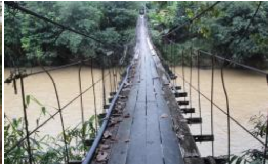
Some railings and timber floor boards were missing from the derelict suspension bridge.
