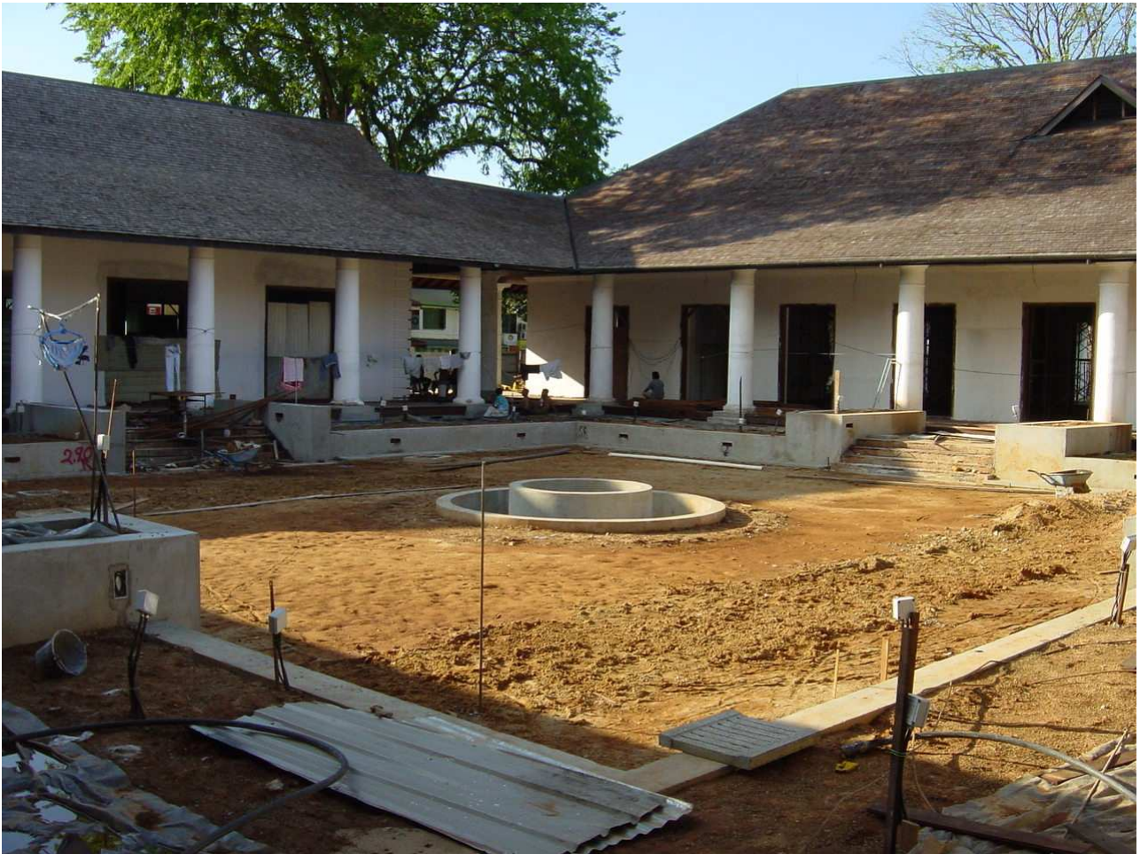
View of the courtyard of the Old Kuching Courthouse during restoration (Copyright John Ting)
